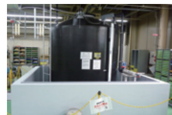
Tank for collecting hydrofluoric acid waste fluid
