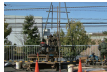
Inspection well for the collection and testing of groundwater
